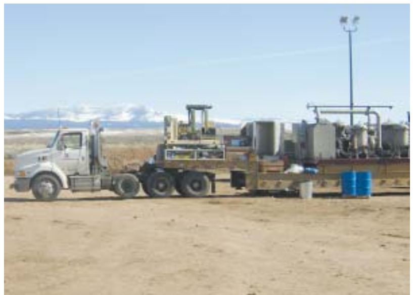
[ABOVE] UPI's high performance lube oil flushing system is easy to set up virtually anywhere. This on the job photo shows work being done in California.
